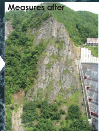
The rockfall protection wire nets which covers the base rock slope
